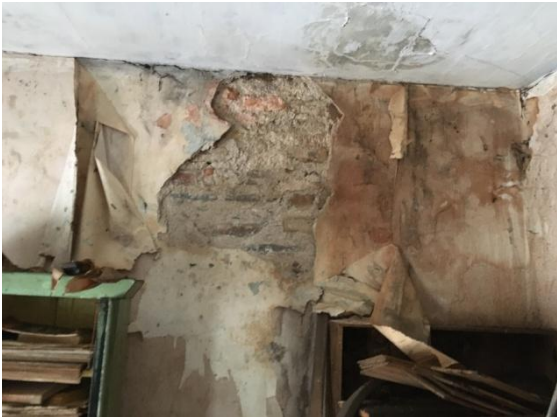
Fig.51; Top-floor, wall adjacent to no.23 Thomas Hill.
