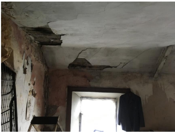
Fig.45; Top-floor, damp ingress through ceiling and walls.
