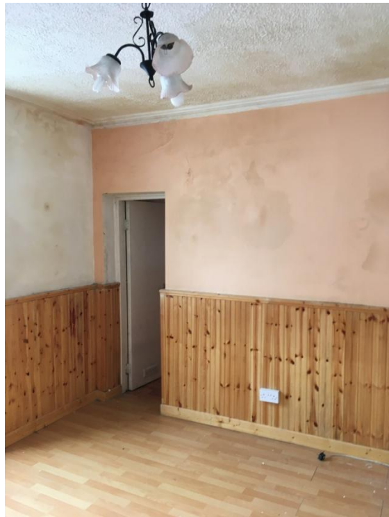
Fig.26; Extreme damp, and door to side-room which stands adjacent to the higher-level Queens Terrace
