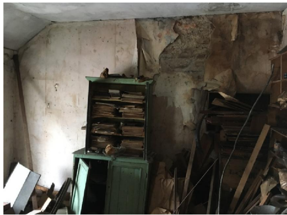
Fig.46; Top-floor, wall adjacent to no.23 Thomas Hill.
