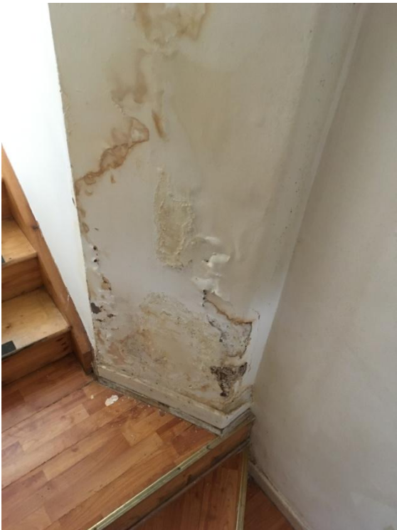
Fig.15; Severe damp at mezzanine-level.
