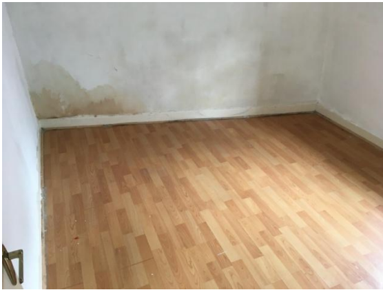
Fig.1; Damp to end gable-wall at second-floor level.
