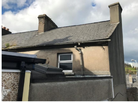
Fig.38; Defective gutters, asbestos tiles, missing render.
