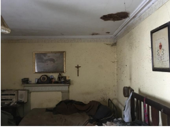
Fig.55; First-floor; original features, damp and stains
