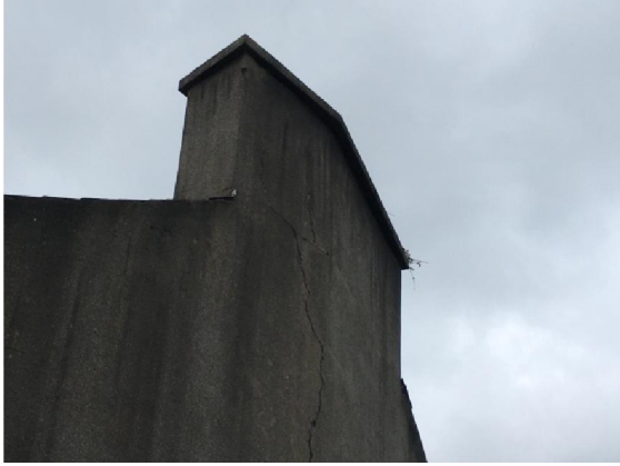
Fig.37; Significant crack in end gable to Queens Trc.
