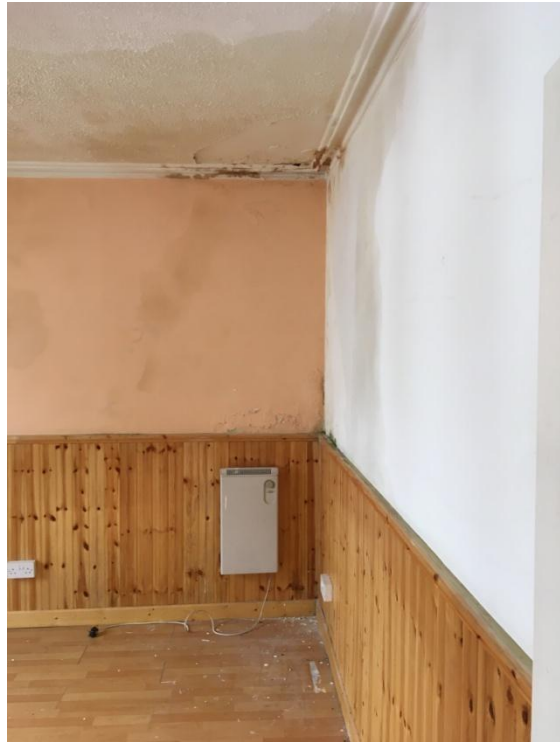
Fig.24; Ground-floor, front room; extreme damp ingress.
