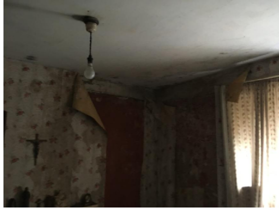
Fig.56; Damp walls causing wallpaper to peel off.
