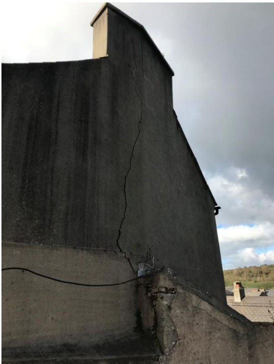
Fig.35; Significant crack in end gable to Queens Trc.
