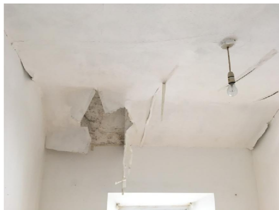
Fig.4; Ceiling at the top of stairs, showing damp ingress.
