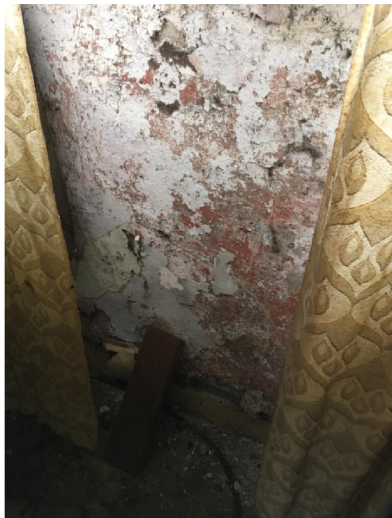
Fig.48; Damp ingress on front wall between windows.
