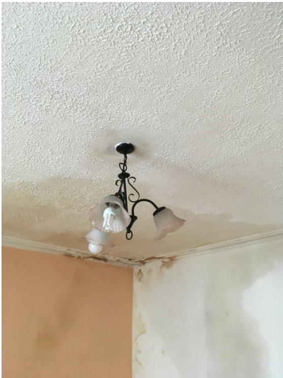
Fig.25; Ground front-room; extreme damp ingress.
