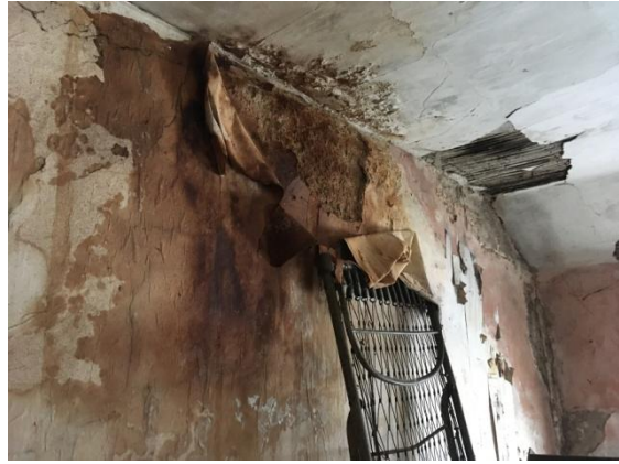
Fig.44; Top-floor, wall adjacent to no.21 Thomas Hill.
