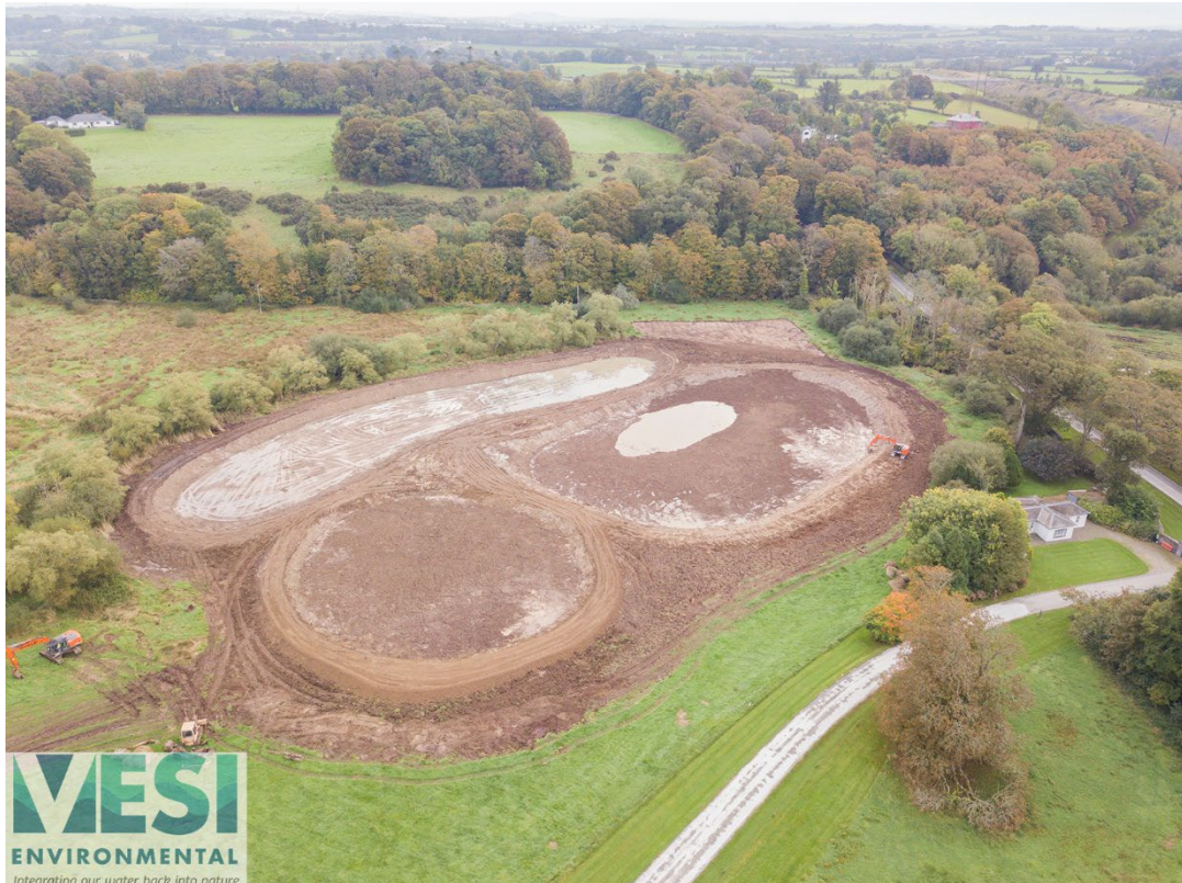
Mount Congreve Integrated Constructed Wetlands
