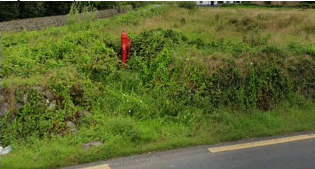
Image 2. Water Pump to be retained
