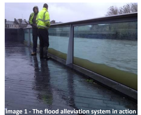
Image 1 - The flood alleviation system in action
