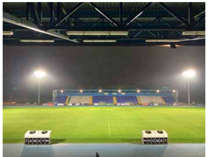
Floodlights installed at the RSC
