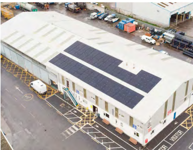
Solar Photovoltaic installation at the WCCC Dungarvan Depot
