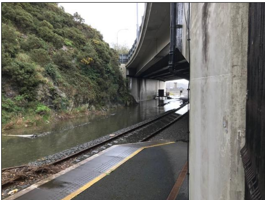
Plate 16.3 Flooding at the Plunkett Station in October 2020
